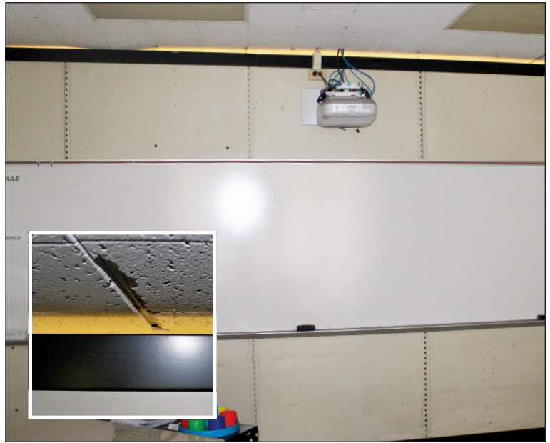
Classroom partition walls, showing gap between ceiling and wall
