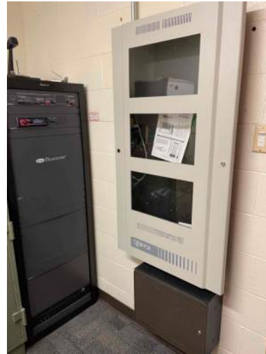
New Fire Alarm Control Panel
